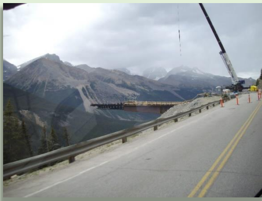
Tour coach view of the Glacier Sky Walk under construction and projecting across the viewscape of the Icefields Parkway. P. Duck Photo
