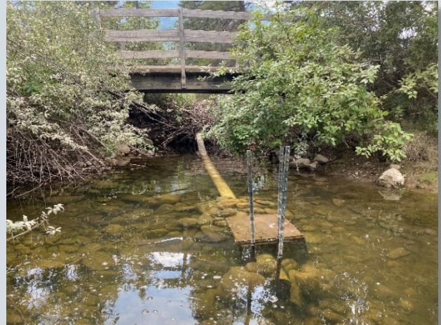
A beaver dam in the background was lowered and this 8-inch pipe with control valve (inside box) was installed during migratory bird nesting season to lower water levels in the Cave and Basin Marsh. The pipe was not installed as prescribed in the environmental impact assessment. A fundamental ecological process was interrupted and manipulated to protect the Town of Banff Recreation Grounds, which have been landscaped to accommodate flooding, from flooding. (P. Duck photo.)
